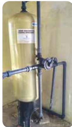
Iron Removal Unit at Government Primary School in Reshalpur, Madhya Pradesh
