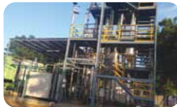
Multi-effect Evaporator at Bosch, Rajasthan
