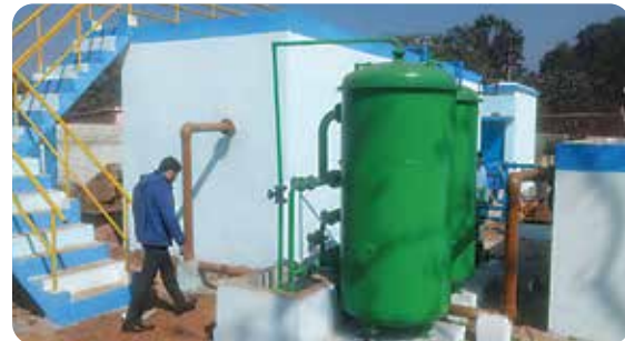
A Section of Fluidised Media Reactor in Keonjhar District Installed for Tata Steel Rural Development Society
