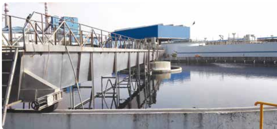
High Rate Solids Contact Clarifier
