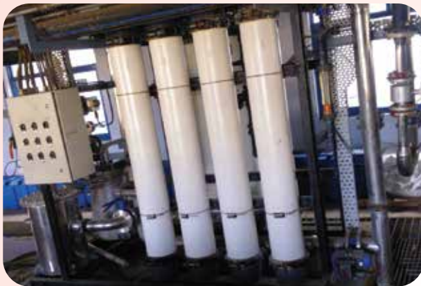
500 m 3 /day Recycle, Ultra Filtration and Reverse Osmosis Plant
