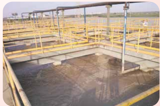
300 m 3 /day Effluent Treatment & Recycle System
