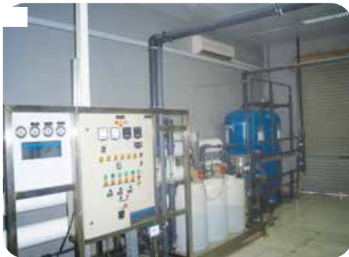
Reverse Osmosis Plant at Coca Cola, Bahrain
