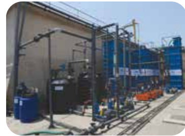
Sewage Recycle Plant using INDION IPC-MBR at Navi Mumbai Municipal Corporation
