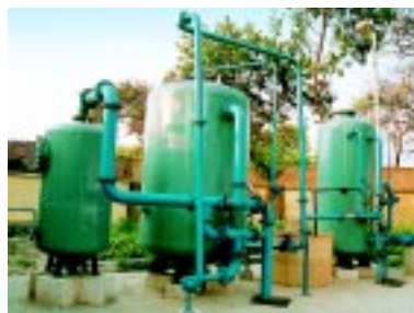
45 m 3 /h iron removal and softening system at Military Engineering Services' Dumayun Army Housing Complex, Garden Reach, Kolkata.
