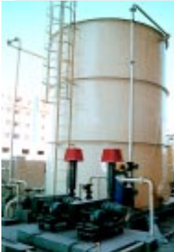
200 m 3 /day fluidised media reactor (inset) and tertiary treatment at Satyam Computers office complex. Sewage is oxidised in the tank to reduce BOD. Tertiary treatment recycles waste water for toilet flushing and gardening.
