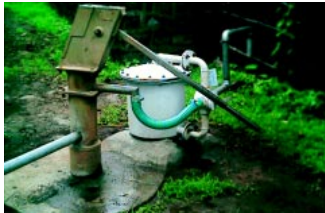
INDION Handpump Attachment for Iron Removal installed at Tondsure.
