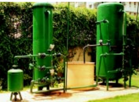
Installed at premier housing properties in Kolkata – iron removal filtration system, 8 m 3 /h, for Mani Group, and iron removal and softening system, 8 m 3 /h, for MK Jalan Properties.
