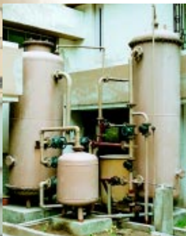
15 m 3 /h iron removal and softening system at Tolly Residency Housing Society, Kolkata.
