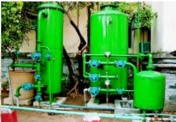
25 m 3 /h iron removal and softening system at Middleton Mansion Housing Society, Kolkata.
