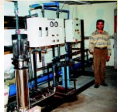
5 m 3 /h RO system for drinking and other applications, caters to the 180 flats in Shakti Apartments, Dwarka.
