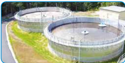
INDION Sequencing Batch Reactor (SBR)
