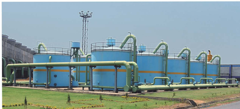
Side Stream Filters at Steel Facility
