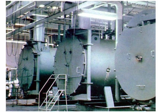
Boiler Water Treatment
