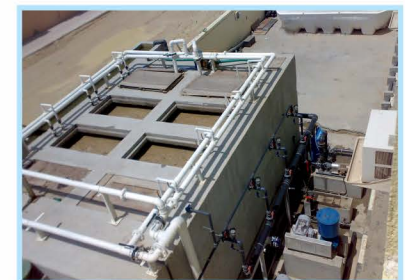
Membrane Bioreactor at Commercial Complex
