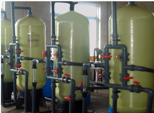
Arsenic Removal Plant for Ground Water Treatment
