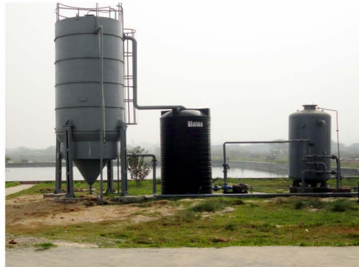
Continuous Sand Filter for Surface Water Treatment
