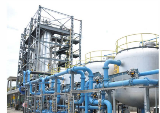
Zero Liquid Discharge System at Synthetic Rubber Plant
