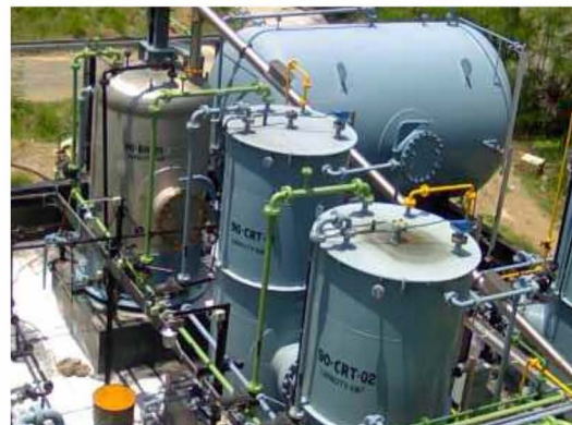
Boron Enrichment Plant for Heavy Water Board
