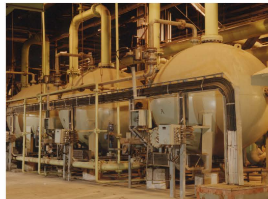
Condensate Polishing Units for Power Plant
