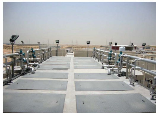
Membrane Bioreactor Plant at Industrial Area
