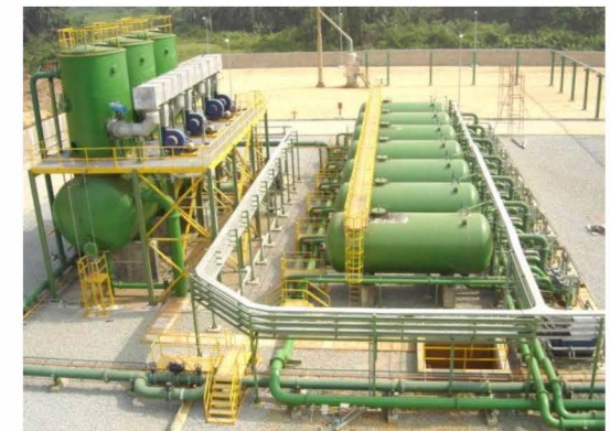
Filtration System at Power Plant
