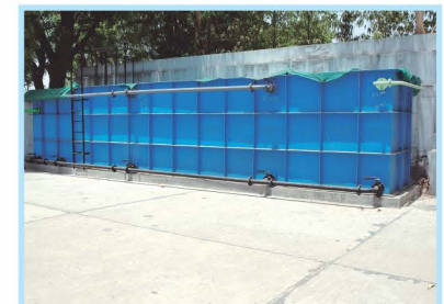
Fluidised Media Reactor at a Hotel
