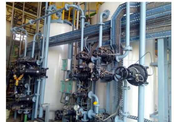
Glycol Purification for Chemical Plant
